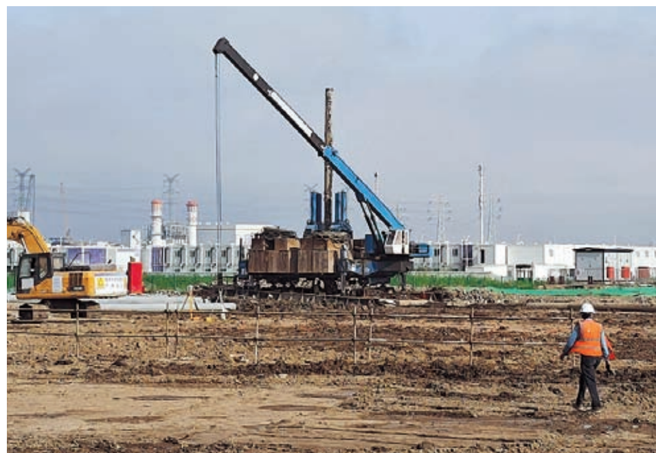
A view of the construction site of Tesla's new mega factory in the Lingang Special Area of Shanghai. — Sun Minjie
